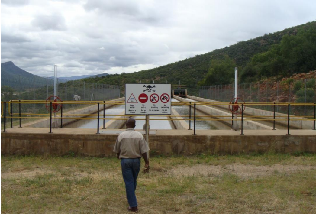
Figure 1: View from outlet end towards inlet end of Lebalelo Weir Desilting Works (example)
